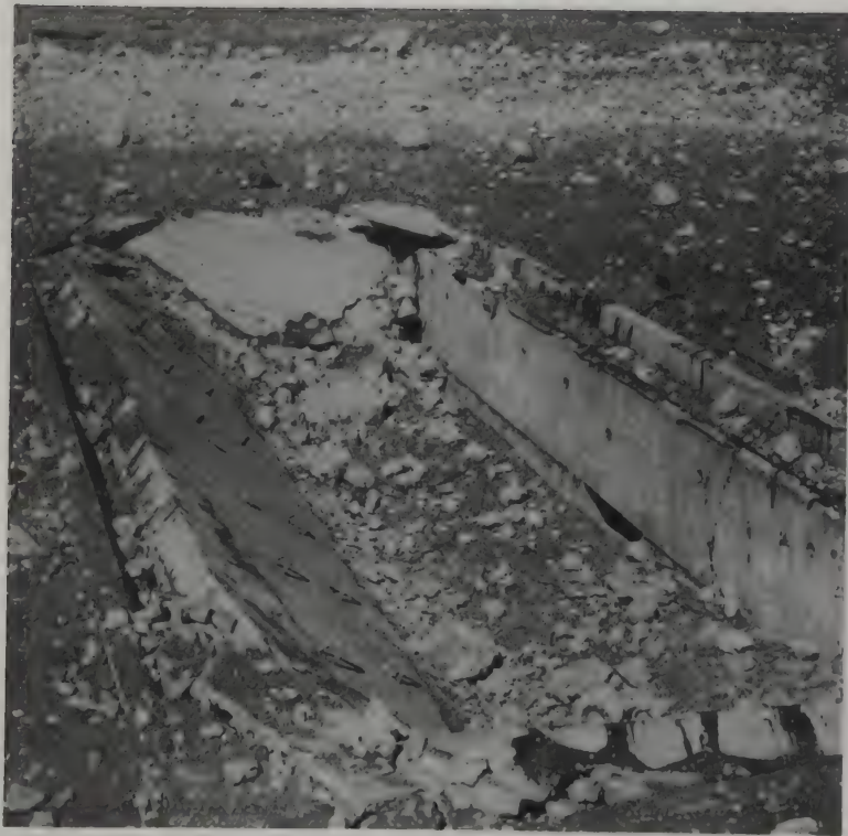
FIG.18. DAMAGE TO FULL SCALE PANEL AT 21.6 PSI.
